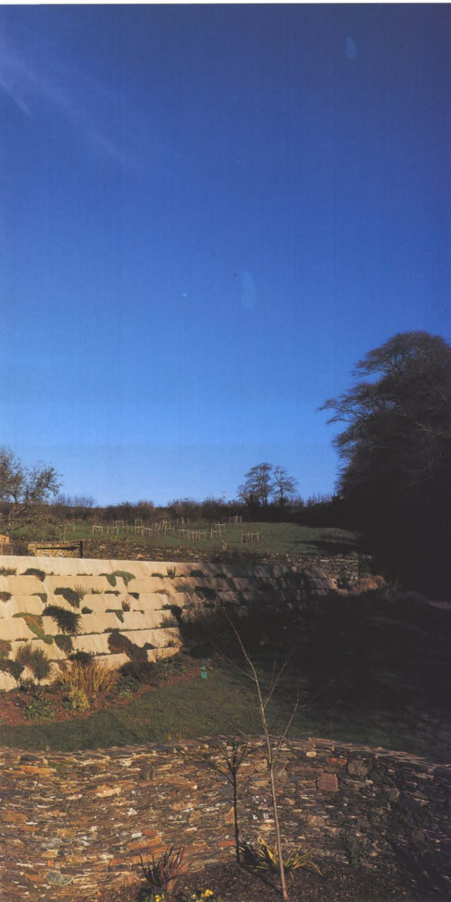
2. The lawn is retained by precast-concrete stepped slabs forming a planted wall
